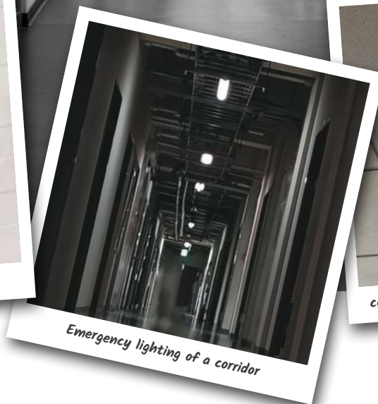
Wall mounting of the emergency light
